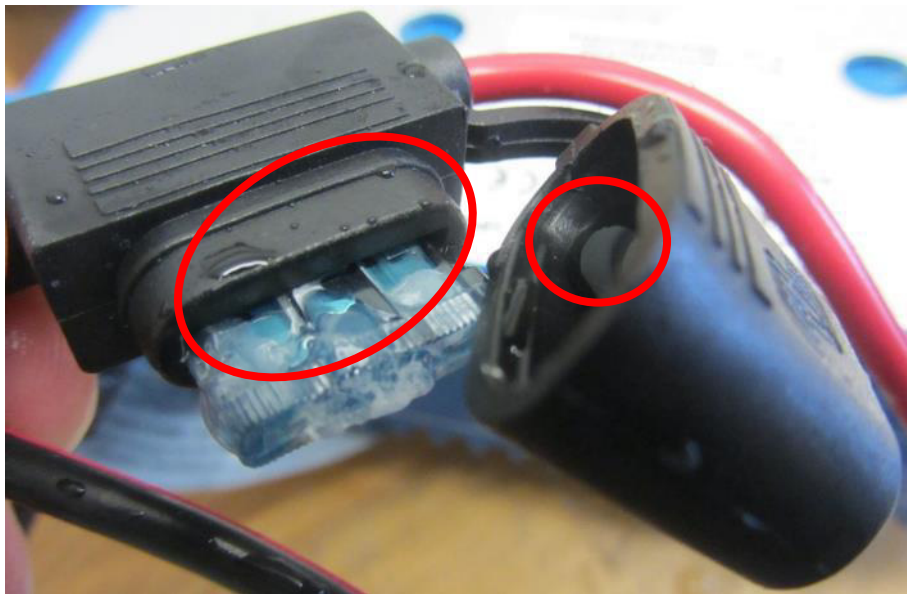
Figure 21: Detailed view of water drop in the fuse box of Sample B after Method of Test—Sealed Devices
